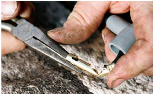
6 Prior to crimping on the connector, we slid the 90-degree boot onto the wire (with the help of a little WD-40). The connector is designed with a relief to easily bend to 90 degrees with the help of a pair of needle-nose pliers. Then the boot slid down over the connector and pushed into the appropriate contact on top of the distributor cap.
